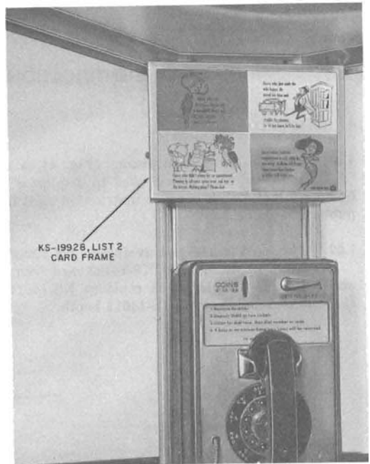
Fig. 3 — KS-19928, List 2 Card Frame Mounted in Corner of Telephone Booth
