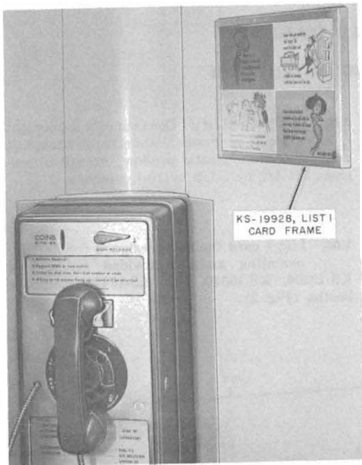
Fig. 2 — KS-19928, List 1 Card Frame Mounted on a Flat Wall
